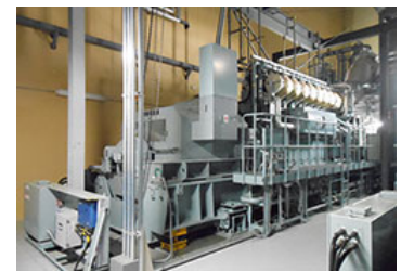
Gas engine powered CGS
