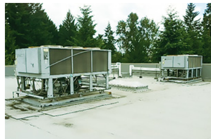
Air conditioning system installed on the roof
