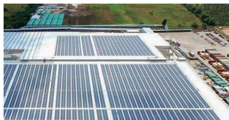
New factory in the Philippines with a rooftop mega-solar power plant with a maximum output of 3,000 kW of power (2017)
